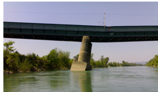
The railway bridge Jakuševac in Mičevac on the Sava River that collapsed on March 30, 2009
